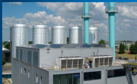
Energy and process cooling
