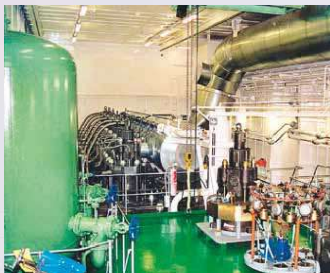
Ship engine cooling
