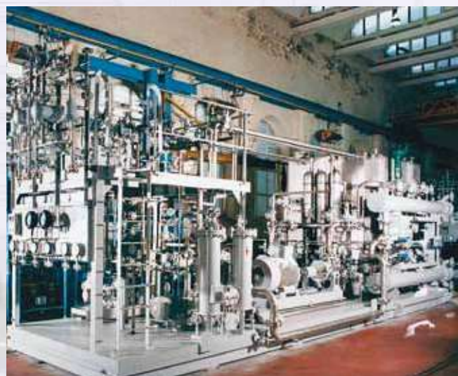
Compressed air cooling
