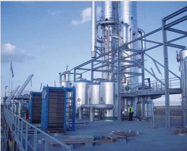
Condensation of bioethanol.
